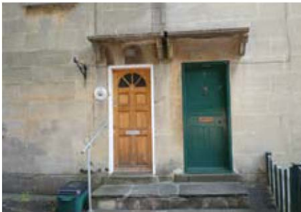
Ivy Cottages form an attractive terrace of locally important buildings that have undergone insensitive alterations that have had a negative impact on their appearance such as inappropriate modern replacement doors and windows. The door on the right of the photographs is the original door.
